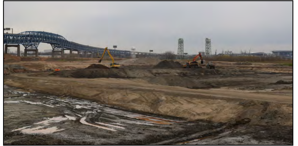
Diamond Materials LLC removes dredged sediment from the Fort Mifflin Dredged Material Placement Facility, owned and operated by the U.S. Army Corps of Engineers. The sediment will be beneficially used for development in Morrisville, New Jersey. (Photo by Kat Tracey)
